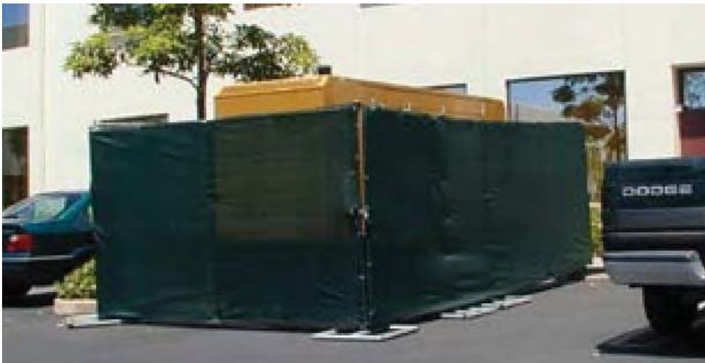
Figure 5-26 Example of Inappropriate Ground Mounted Equipment Screening
