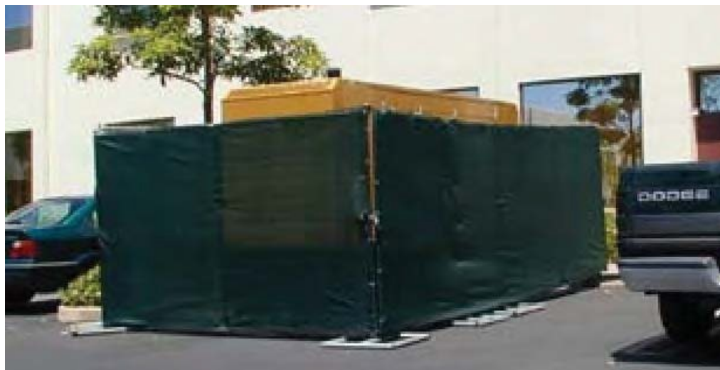
Figure 5-26 Example of Inappropriate Ground Mounted Equipment Screening
