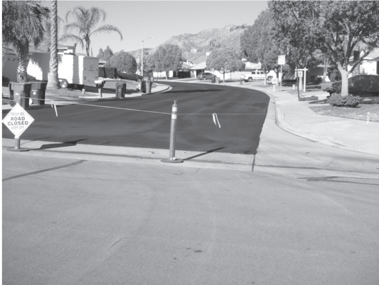
Slurry Seal Program Zone II (Selected Streets) Deercreek Rd at Sycamore Canyon Rd Shown Above
