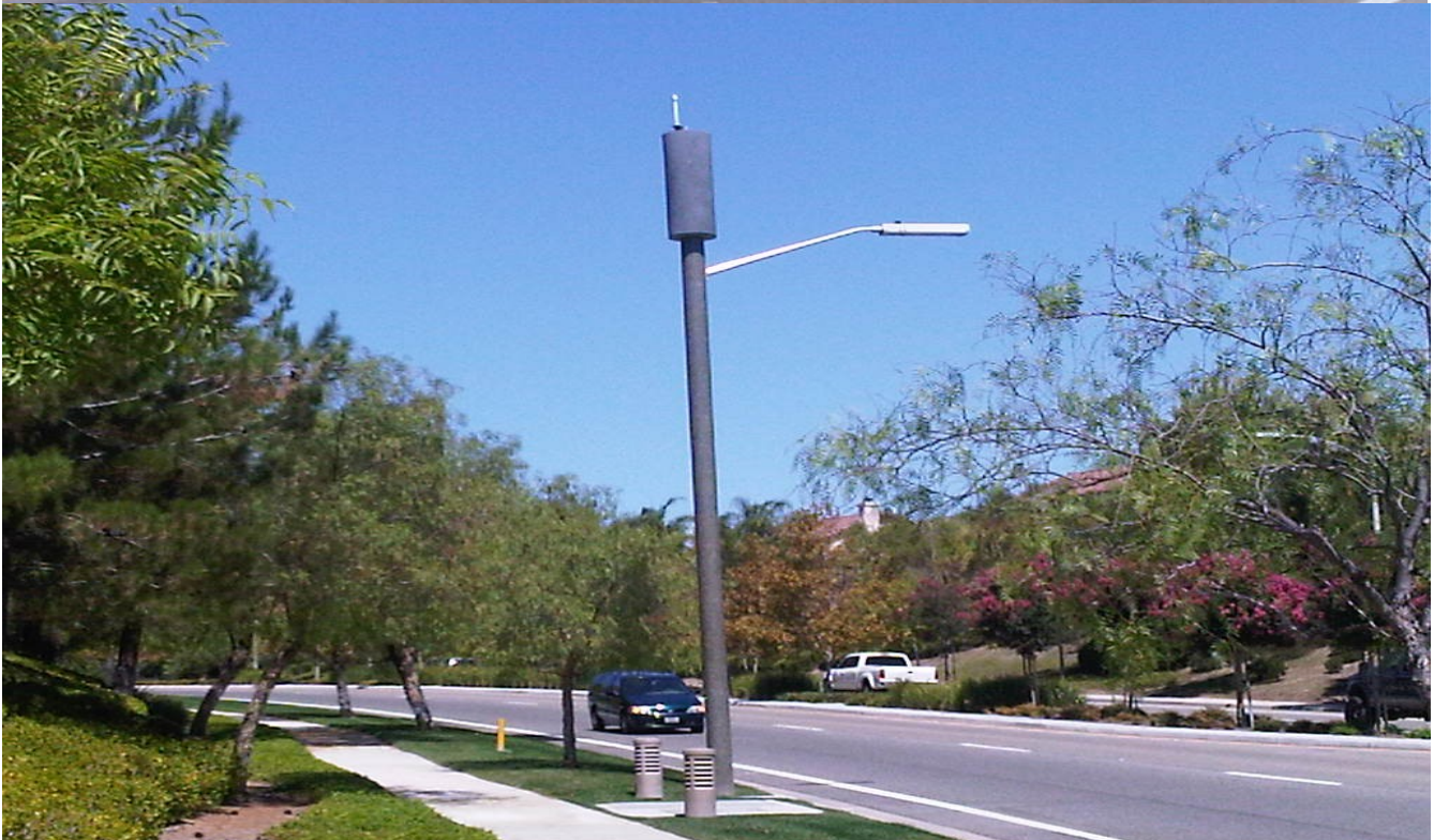
Example T-Mobile/Southern California Edison Street Light Pole
