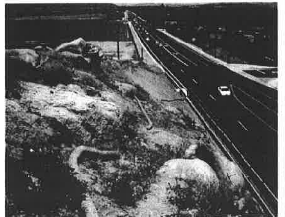
Loren was Leighton’s Senior Engineering Technician for geotechnical field observation and compaction testing on the City’s Lassalle Street Widening project.
