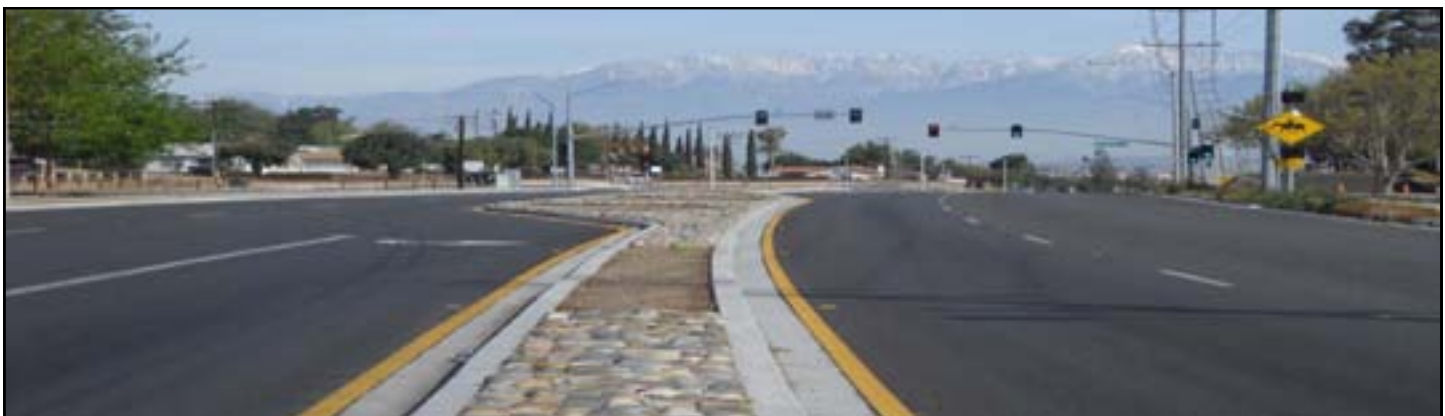
Hamner Avenue widening Project from Sixth Street to Detroit Street, City of Norco (Photo courtesy of City of Norco)
