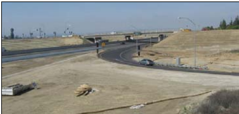
Nason / SR-60 Interchange Project, City of Moreno Valley (Photo courtesy City of Moreno Valley)
