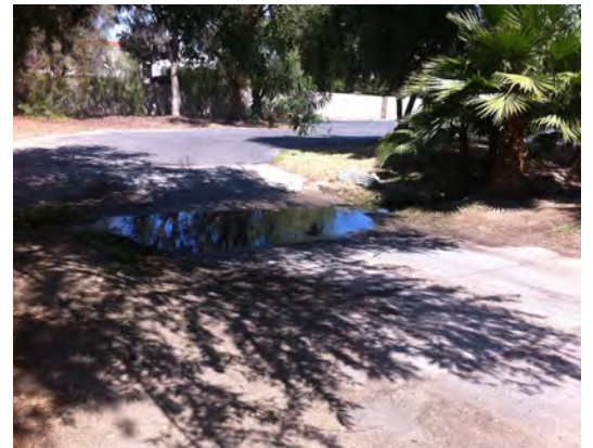
Poor drainage at low point in apartment complex.
