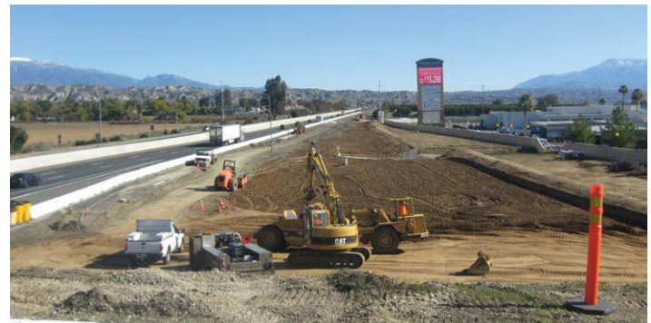
Moreno Beach Drive / SR-60 Interchange Project, City of Moreno Valley. (Photo courtesy City of Moreno Valley)
