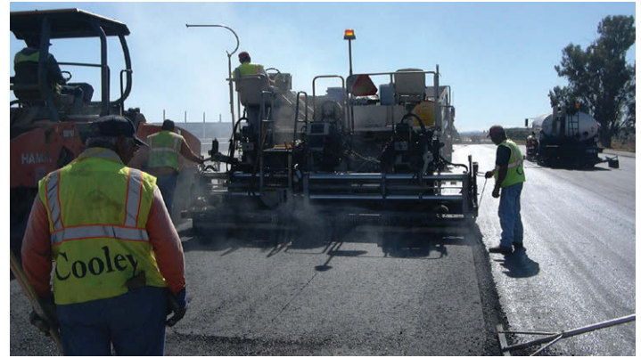
Heacock Street, Perris Valley Storm Drain to San Michele Road Widening Project, March Joint Powers Authority and City of Moreno Valley. (Photo courtesy City of Moreno Valley)
