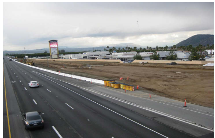
Moreno Beach Drive / SR-60 Interchange Project, City of Moreno Valley. (Photo courtesy City of Moreno Valley)
