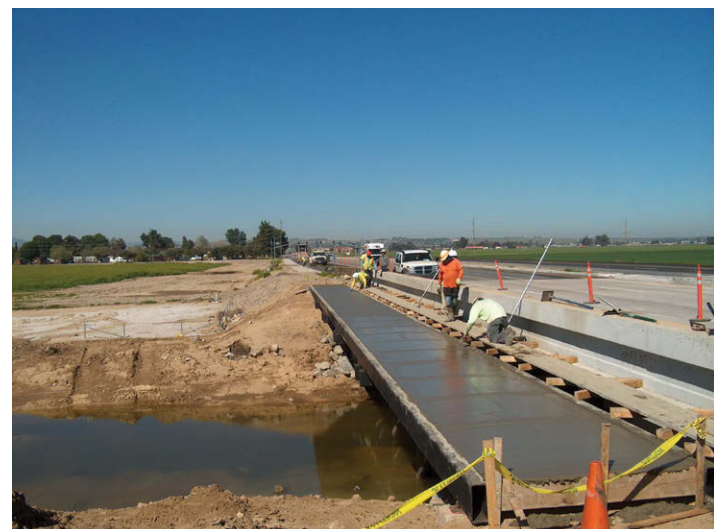
Ramona Expressway Pedestrian Bridge Project, City of Perris. (Photo courtesy Tri Lake Consultants)
