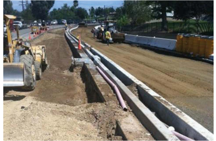
Railroad Canyon Road Widening Project. (Photo courtesy City of Canyon Lakes and Tri Lake Consultants)
