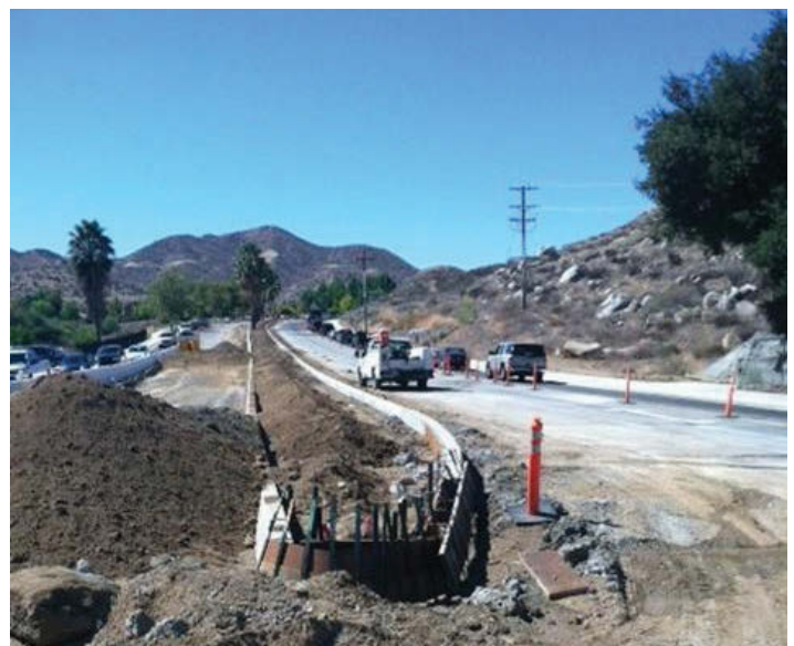
Railroad Canyon Road Widening Project. (Photo courtesy City of Canyon Lake and Tri Lake Consultants)
