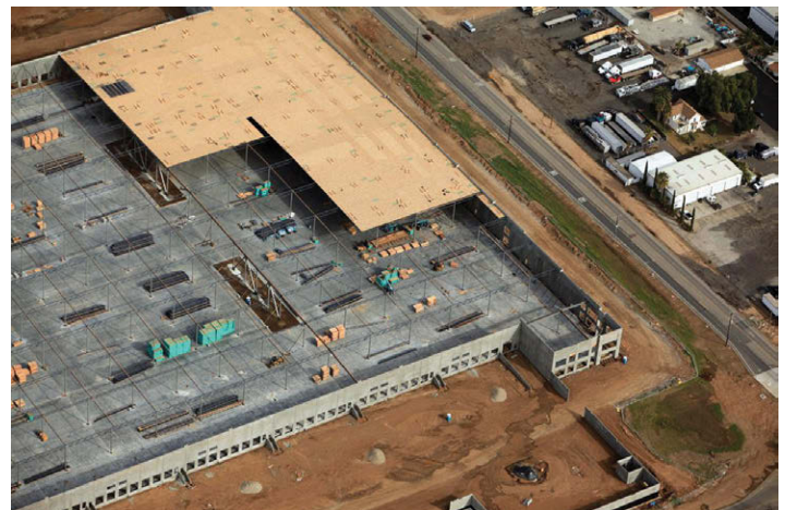
Industrial warehouse construction, City of Moreno Valley. (Photo courtesy of Skyview Imaging)
