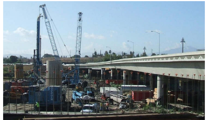
Van Buren Bridges over the Santa Ana River, County of Riverside TLMA. (Photo courtesy County of Riverside TLMA)
