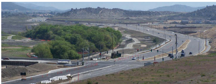
Goetz Road, Newport Road to Murrieta Road Widening. (Photo courtesy of the County of Riverside TLMA)
