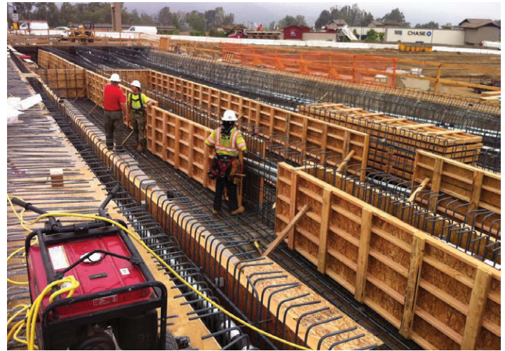
Clinton Keith Road / I-15 Interchange Project, City of Wildomar and County of Riverside TLMA. (Photo courtesy County of Riverside TLMA)
