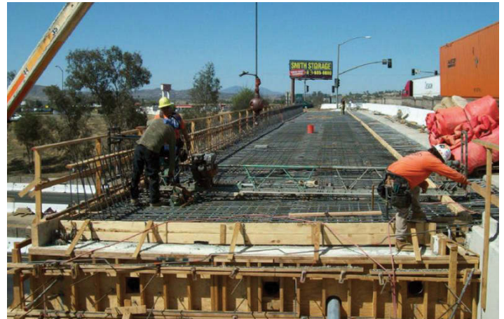
Ramona Expressway / I-215 Interchange Project, County of Riverside TLMA and City of Perris. (Photo courtesy County of Riverside TLMA)
