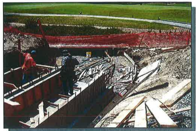
Candleberry Avenue Storm Drain - Double 5-ft. (W) x 3-ft. (H) RCB Outlets to Old Ranch Golf Course Detention Basin
