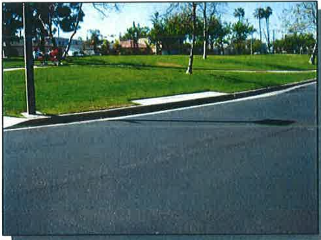
Electric Avenue (north) - Catch Basin Inlet
