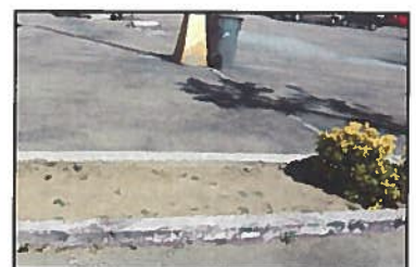
Missing required landscaping and mulch.
