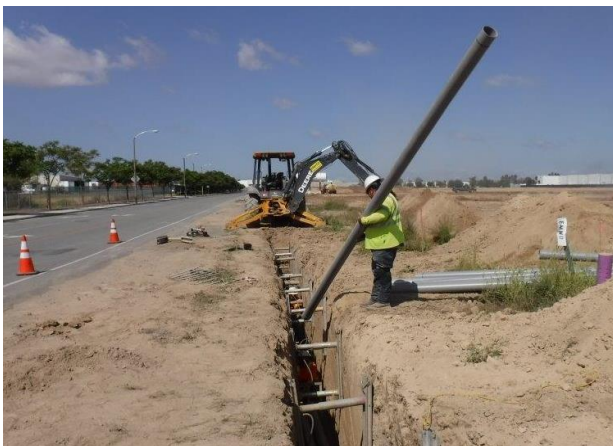
Kitching Substation Feeder Line - Modular 12kV
