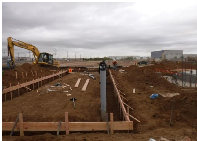
Kitching Substation and SCE Switchyard / Facility Upgrades
