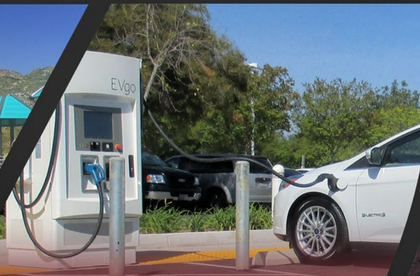
City Hall Electric Vehicle Charging Station
