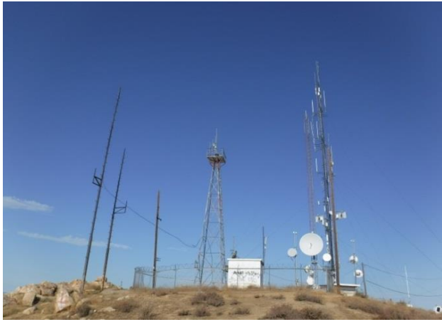
Box Springs Communications Site
