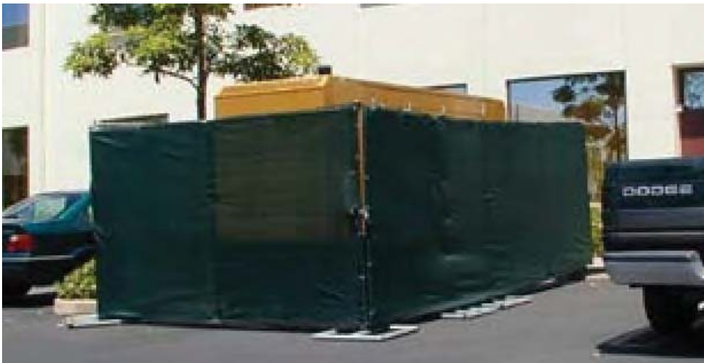
Figure 5-26 Example of Inappropriate Ground Mounted Equipment Screening
