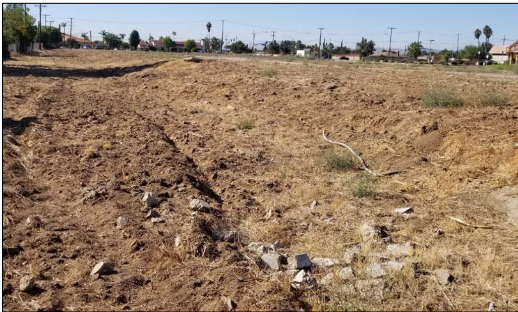
Plate 3. Overview of the berm located along the eastern border of project area, view to the south.
