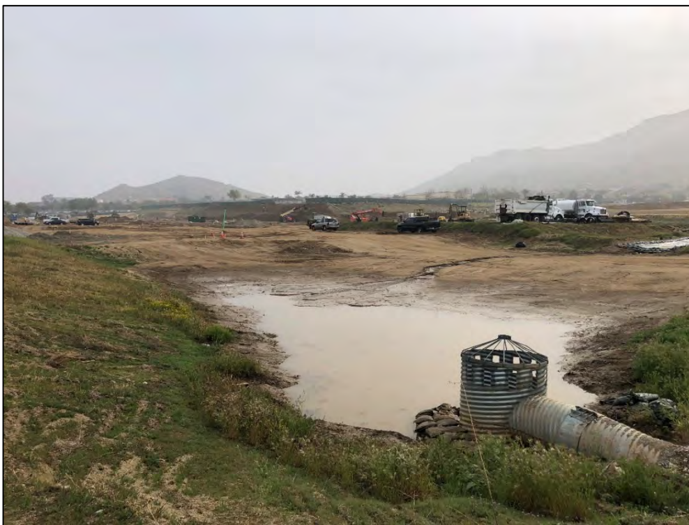
Retention Basin located on the northwestern most portion of the site to capture and retain the nuisance water and runoff.
