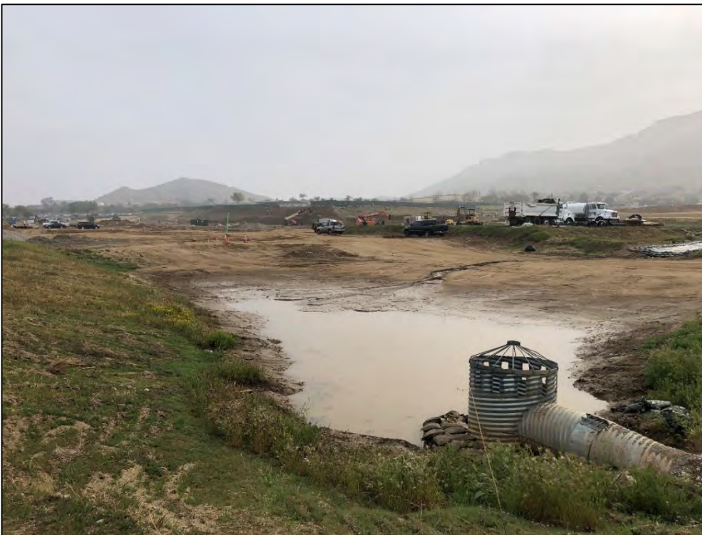
Retention Basin located on the northwestern most portion of the site to capture and retain the nuisance water and runoff.
