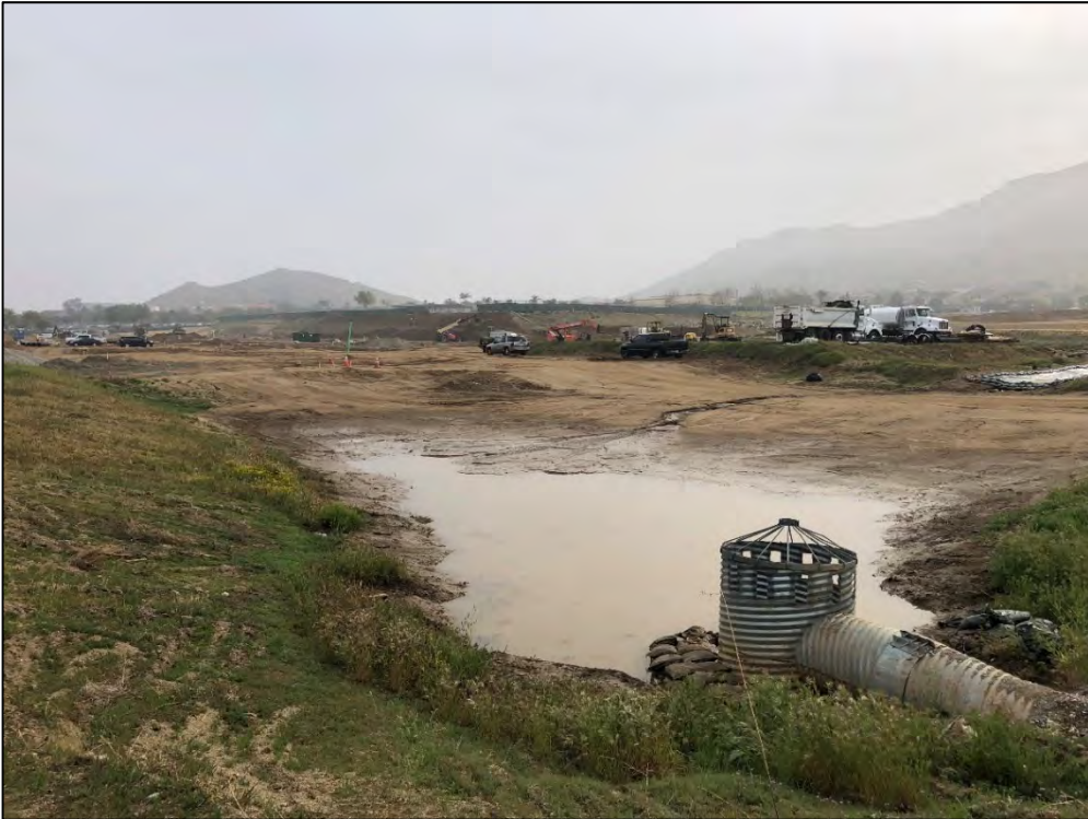
Retention Basin located on the northwestern most portion of the site to capture and retain the nuisance water and runoff.
