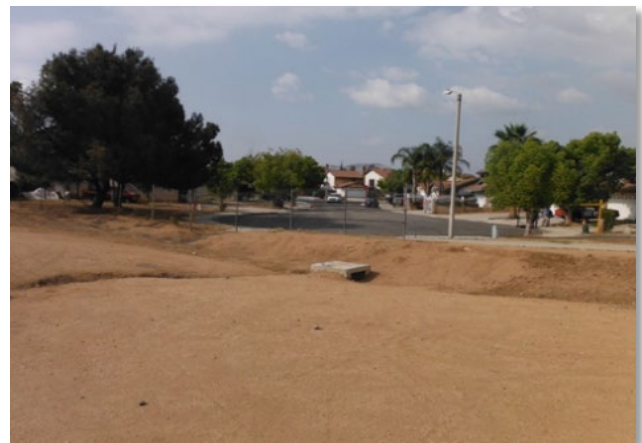
Existing drainage structure between Bay Avenue and Caspian Way to be protected in place.
