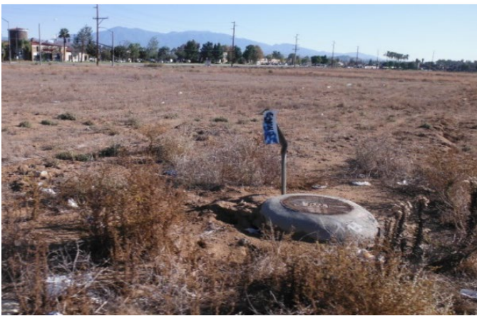
Existing manhole between Alessandro Blvd and Brodiaea Ave, north of Rebecca St.
