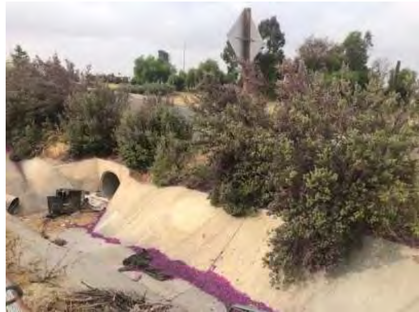
Photo 4. Location where flows leave site into V-ditch - carried off site under 60 freeway and terminate in catchbasin
