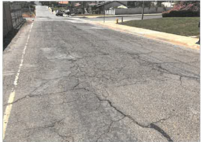
Kalmia Avenue Looking West Limits of Pavement Replacement will be Coordinated with the City
