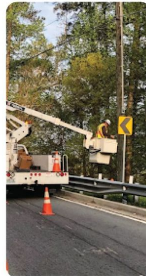
City Foot Traffic Street Electric & existing pole
