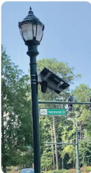
City intersection Solar & existing pole
