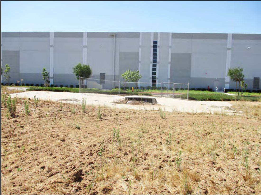
Photograph 2 - Southward view of down drain located at end of the end of Drainage A
