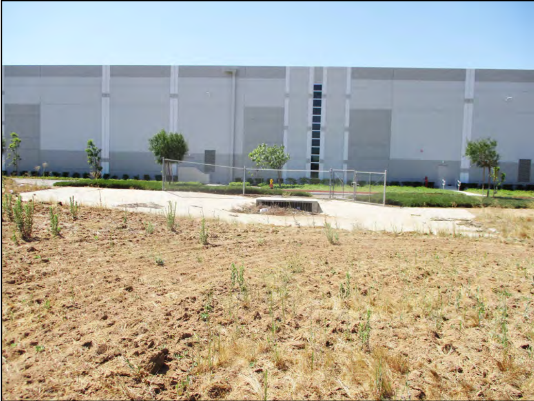
Photograph 2 - Southward view of down drain located at end of the end of Drainage A
