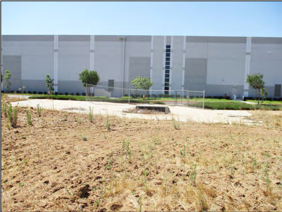
Photograph 2 - Southward view of down drain located at end of the end of Drainage A
