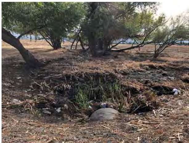
5.View of a storm water drain (easement) draining onto the subject property.
