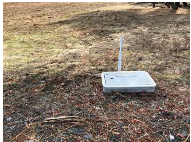
4.View of the communication utility boxes on the north boundary of the subject property.
