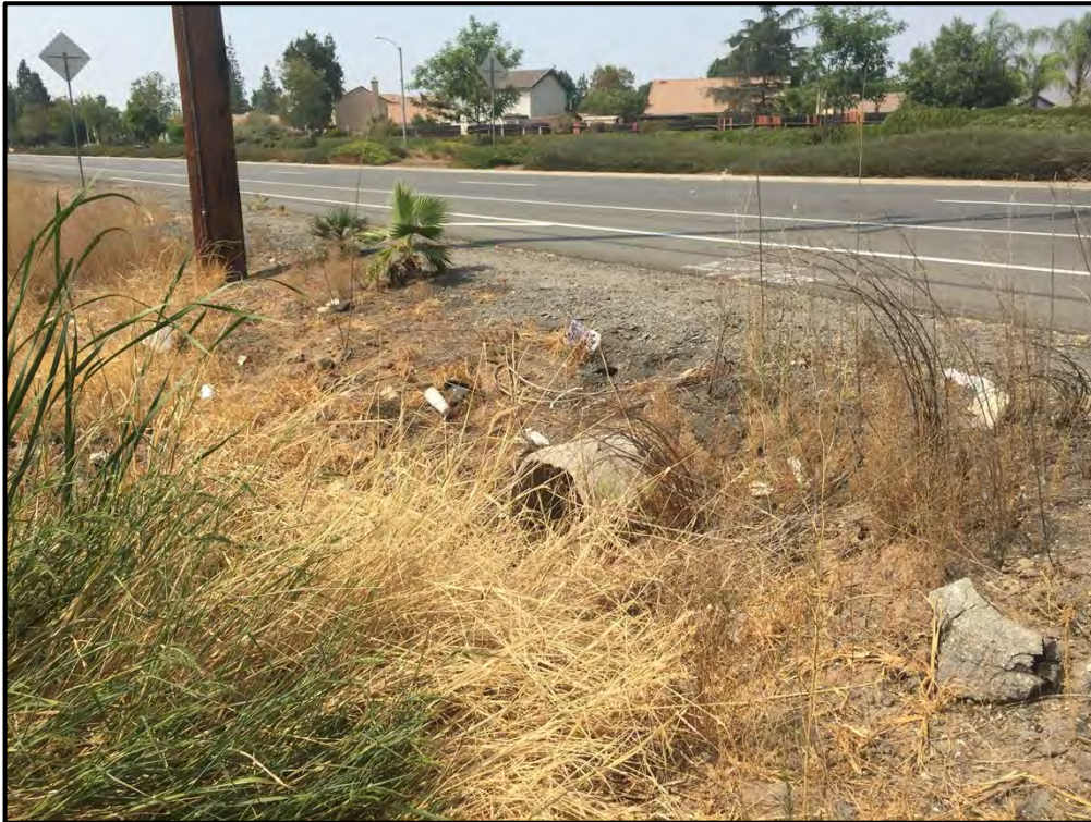
Plate 5.2-3: View of a concrete culvert designed to direct water under Alessandro Boulevard onto the subject property, facing north.
