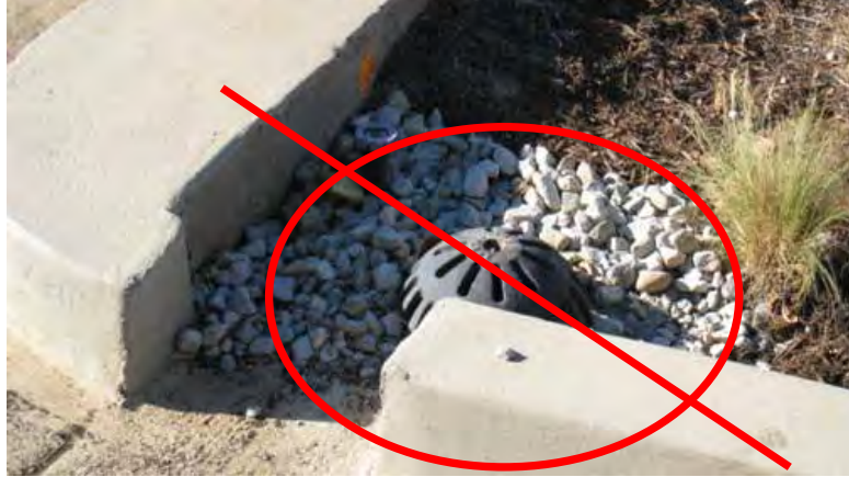
Figure 6: Incorrect Placement of an Overflow Inlet.
