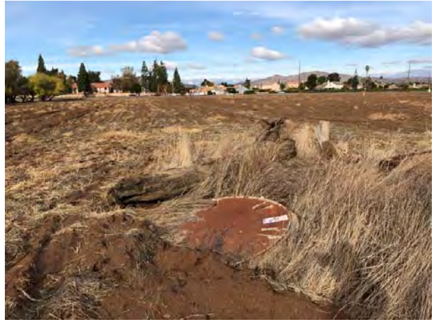
14.View of steel lids abandoned on the south boundary of the subject property.
