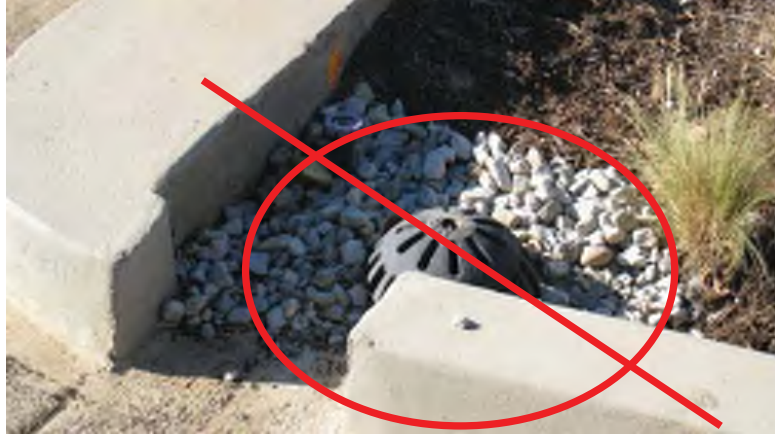
Figure 6: Incorrect Placement of an Overflow Inlet.
