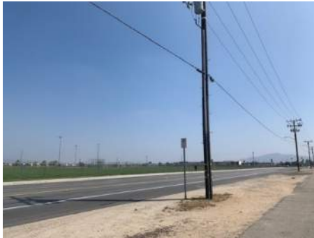
P22- Power Lines in the Northeastern Corners of the Project Site along Iris Ave.
