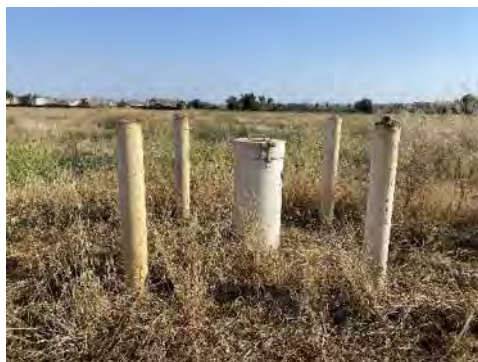
Photo 7: Looking south towards monitoring well: RBMWO3B located along the unpaved portion of Goya Avenue.
