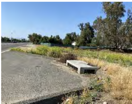
Photo 18: From Indian Street looking north towards an existing drainage inlet along the western boundary of the Project Site.
