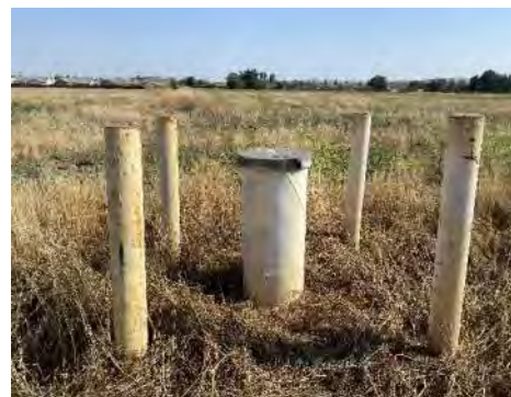
Photo 6: Looking south towards monitoring well: RBMWO3A located along the unpaved portion of Goya Avenue.
