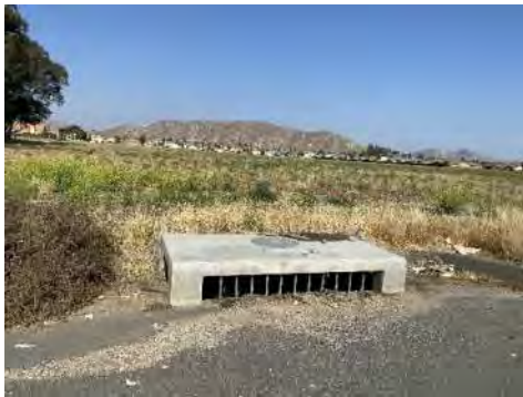
Photo 17: From Indian Street looking east towards an existing drainage inlet along the western boundary of the Project Site.
