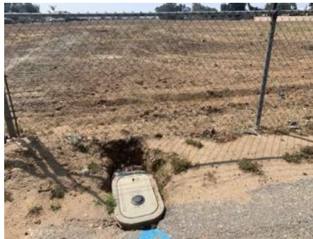
P20- Water Meter on the Northern perimeter of the Job Site on Iris Ave.
